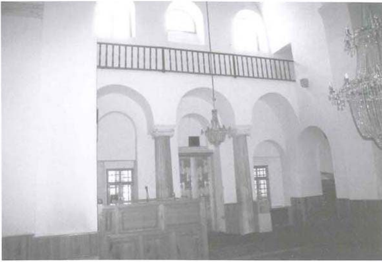
25 North transept of the Panagia Chrysokephalos, Trebizond. The gallery which led from the metatorion to the west balcony is held up on re-used ionic columns. The corbel visible at the east end suggests that the gallery was originally wider
